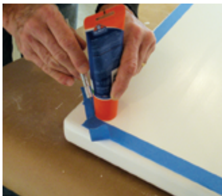
After preparing the surfaces, Stephen masked around the areas to be coated.
